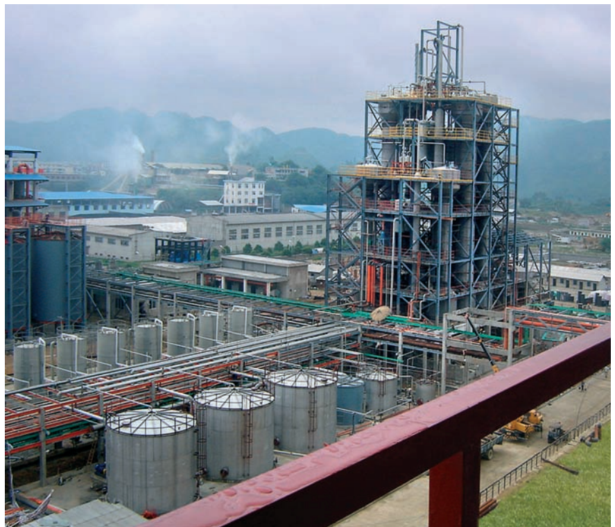
The Wengfu 100,000 t/a purified phosphoric acid plant is China's first to produce PPA from merchant grade phosphoric acid.
